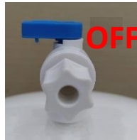
Tank ball valve "OFF"
